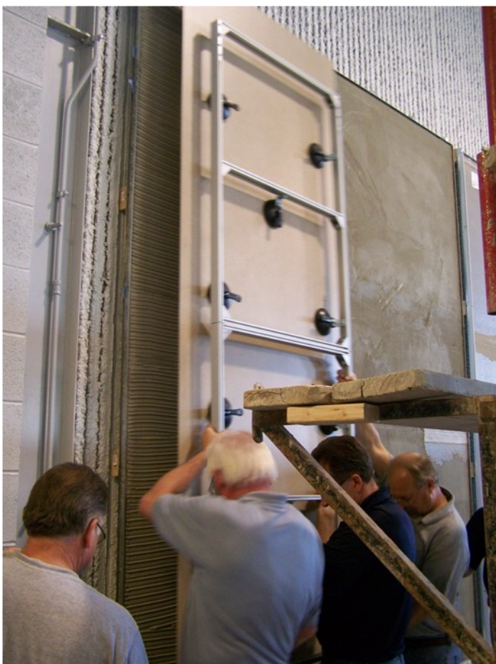
IMI instructors use suction cups to set porcelain wall tile in a setting bed of thinset mortar on cement board.
